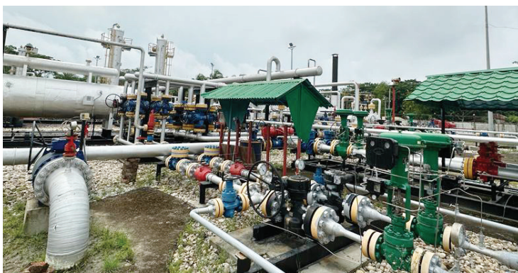
Shahbazpur Gas Field Process Plant
